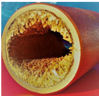
Scale build up on pipe restricting flow
