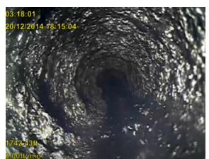
Before CoilHose Intervention
